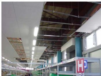
Figure 8. Suspended ceiling damage in an industrial facility after the Japan Niigata Earthquake 2007 [17].
