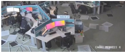
Figure 5. Turkey 2023 Kahramanmaraş earthquakes, suspended ceiling damage in Osmaniye 112 Emergency Call Center after the second earthquake
