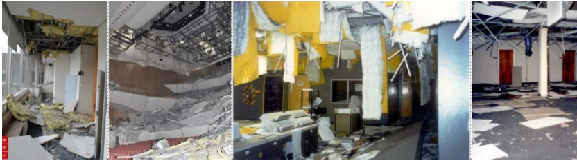
Figure 6. Typical suspended ceiling damages (Url 2).
