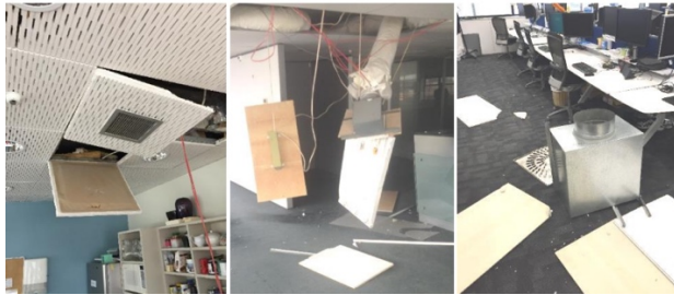
Figure 7. New Zealand 2016 Kaikōura earthquake suspended ceiling system damages [16].
